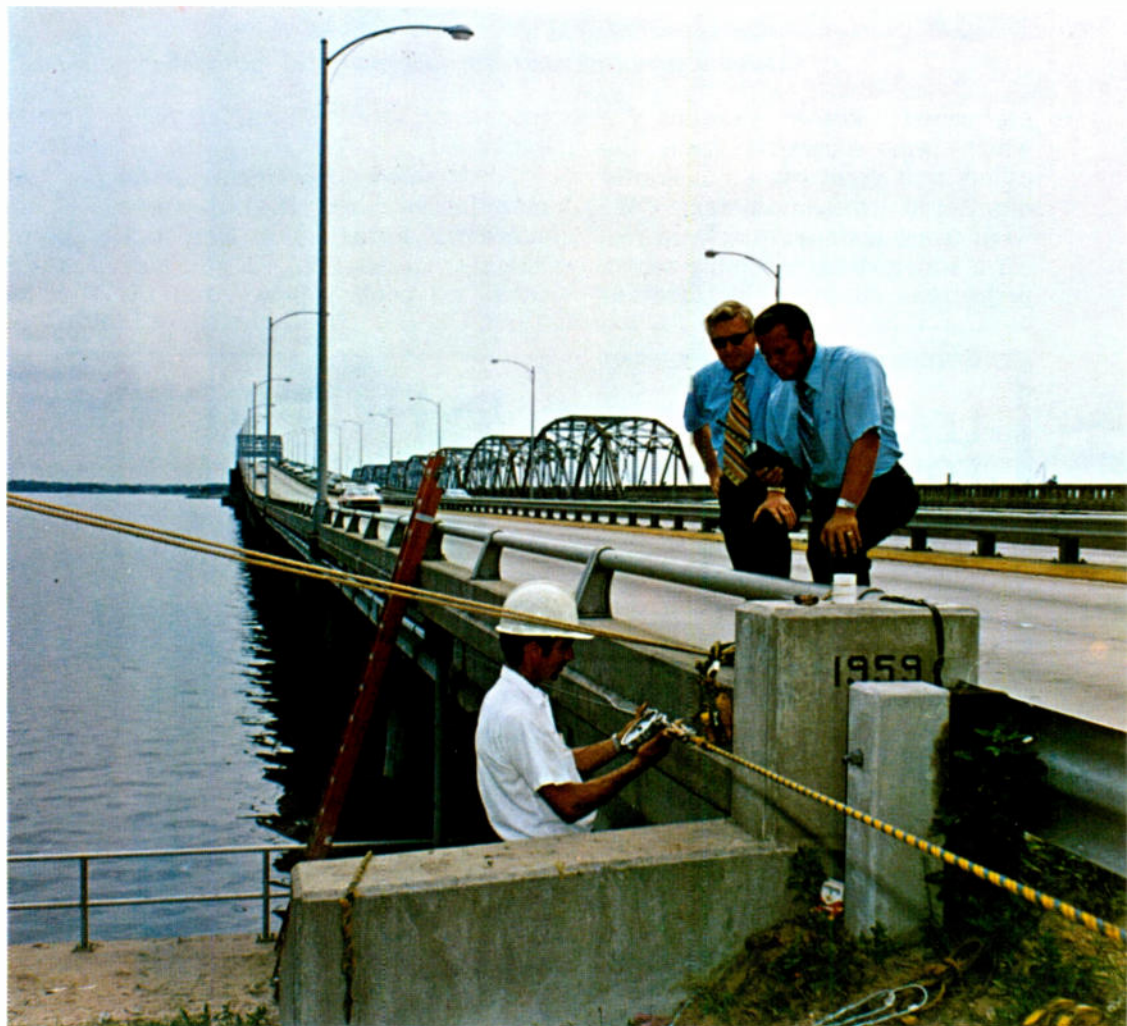
The three-quarter mile cable pull along Hathaway Bridge across Andrews Bay at Panama City, Florida, was coordinated by Clearview Cable TV personnel using two-way radios. Lubricants were liberally applied — continuously — during the unusual cable installation.
