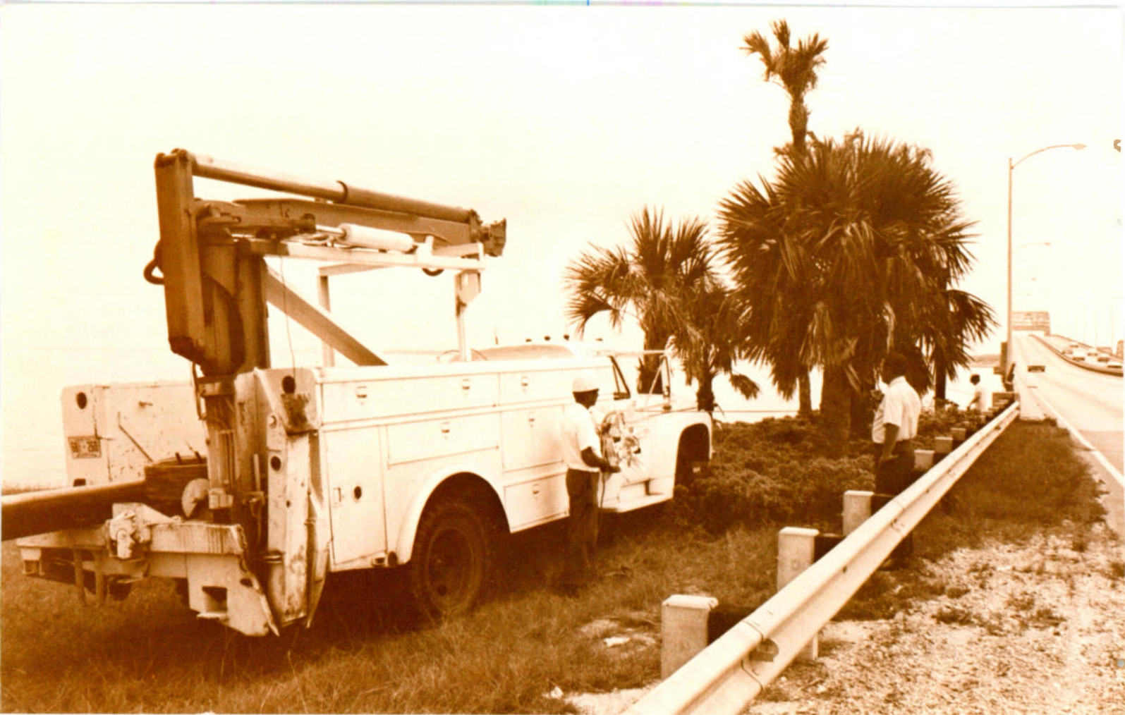
Clearview personnel start the long pull that extended over almost eight hours.
