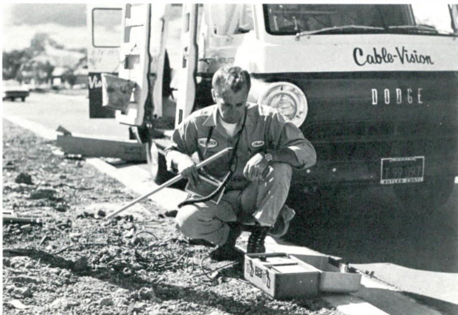
Cable-Vision plant foreman Chuck Christiansen adjusts output signal level on fault locator transmitter. Leads to left are connected with center conductor or shield. Ground lead can be to the unit's ground rod or to pedestal case or anchor bolt on utility pole.
