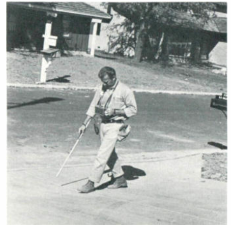
Concrete driveways or streets present no obstacle to tracing cable path. Here, Chuck Christiansen listens to pulsed tone and observes dB intensity meter which provides numerical reference for changes in signal level.
