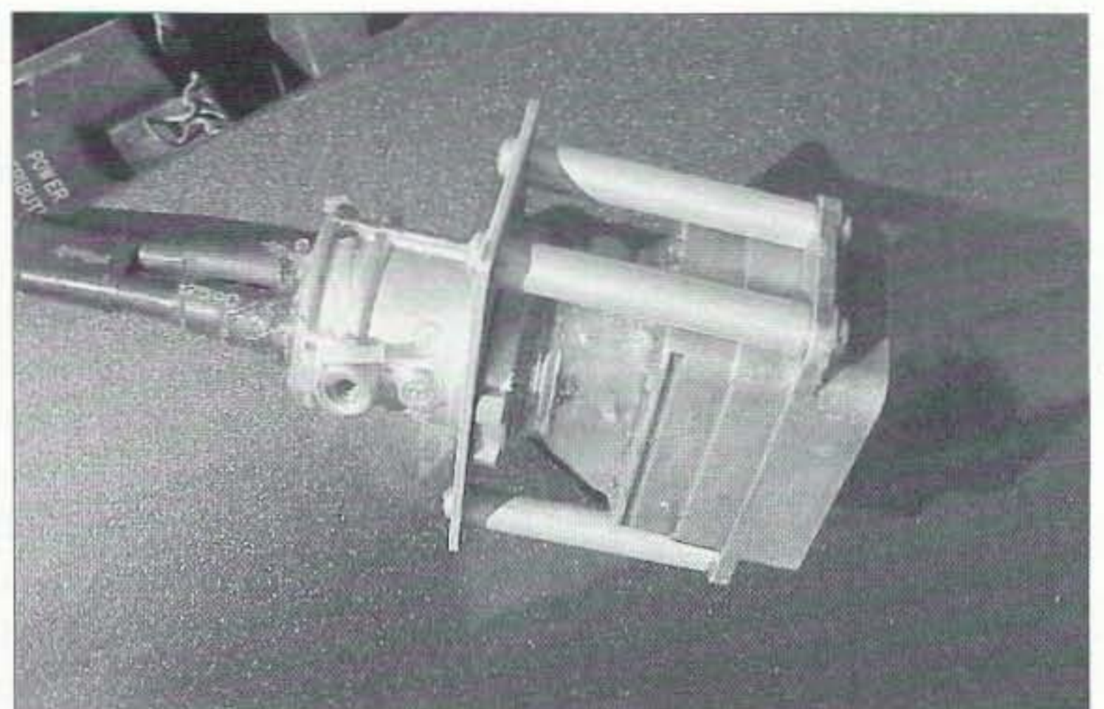
Photo B. Close-up of connector on battery cable. Note homemade backshell consisting of metal stand offs conduit fitting and bathtub sealer.
