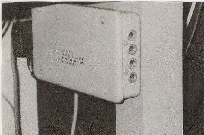
Photo B. The headphone jack box is located on the right table leg.
