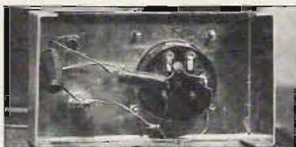
Photo B. Inside the meter. Note the lack of parts.
