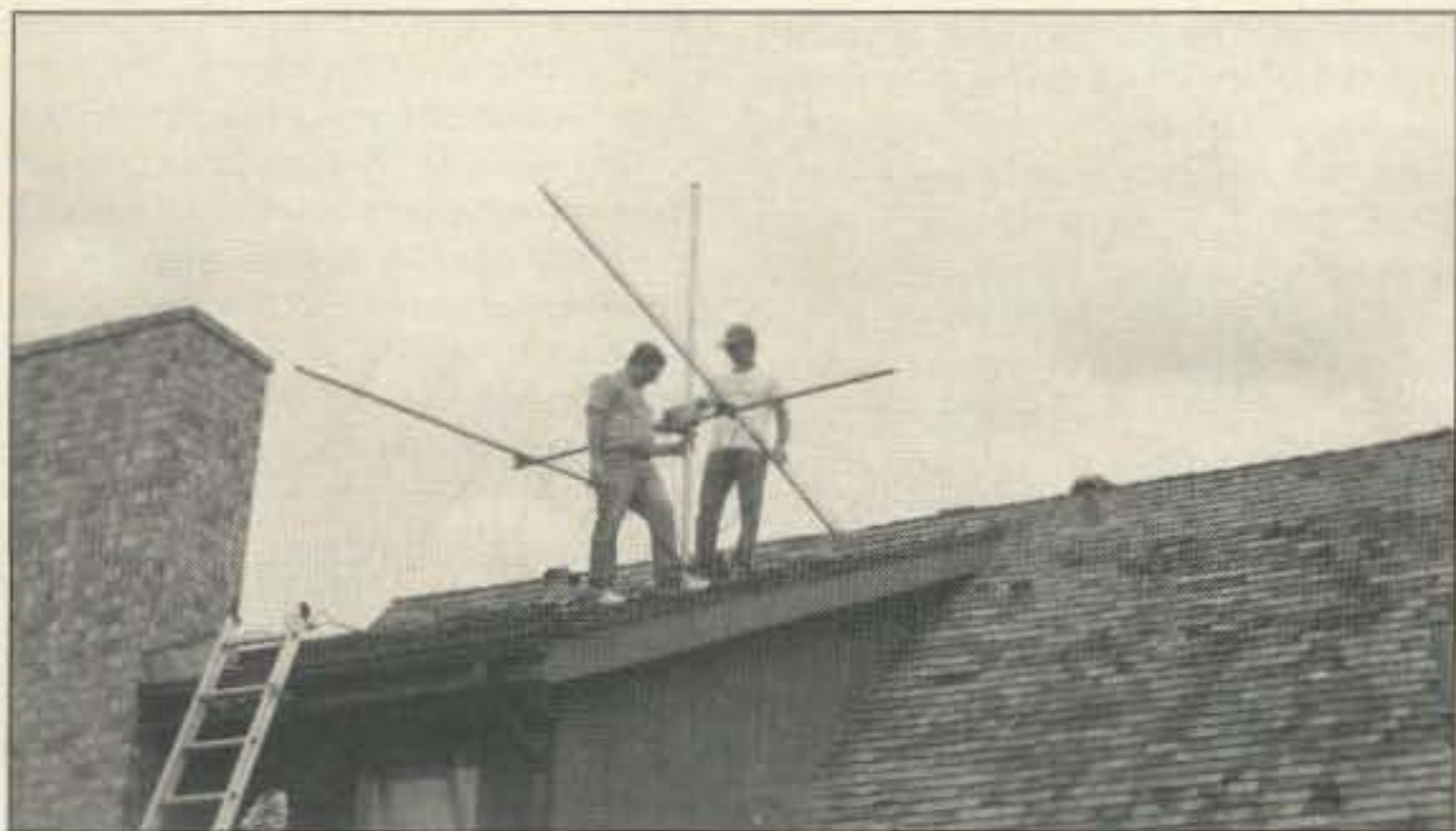
Photo A. WA5WOD and WA5TWT begin installing antennas along the fiberglass boom.
