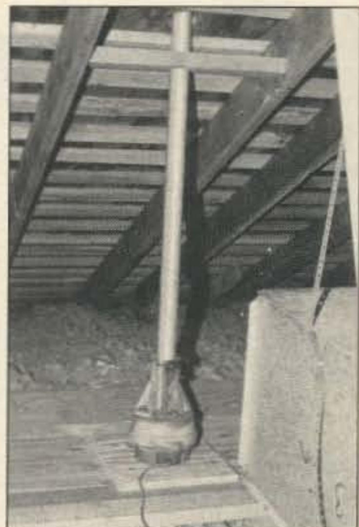
Photo B. The azimuth rotator went in the attic with a 2 x 8 between the rafters for a thrust bearing.
