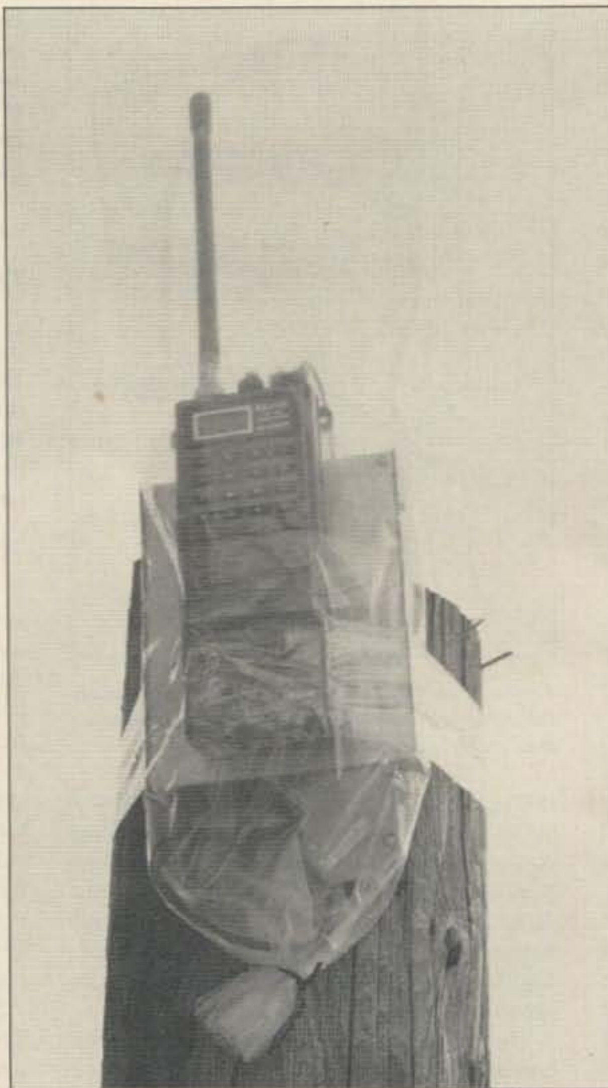
Photo 1. A complete pole-top digipeater with HT and TNC protected with a plastic bag and secured with ducting tape.
