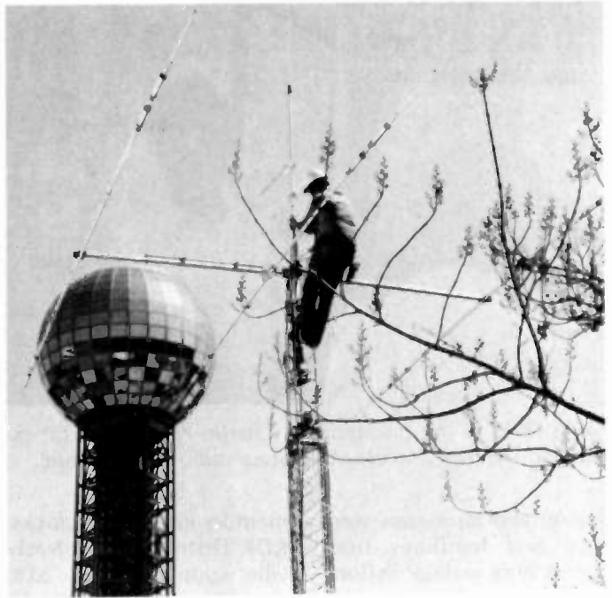
George Child N4BCS installed the 2-meter antenna atop one of the two crank-up towers in the shadow of the Sunsphere.
