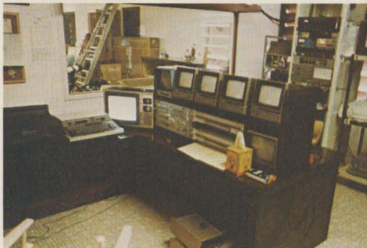
Here are some of the monitors, switching, and other paraphernalia needed to put on a professional television broadcasting service.
