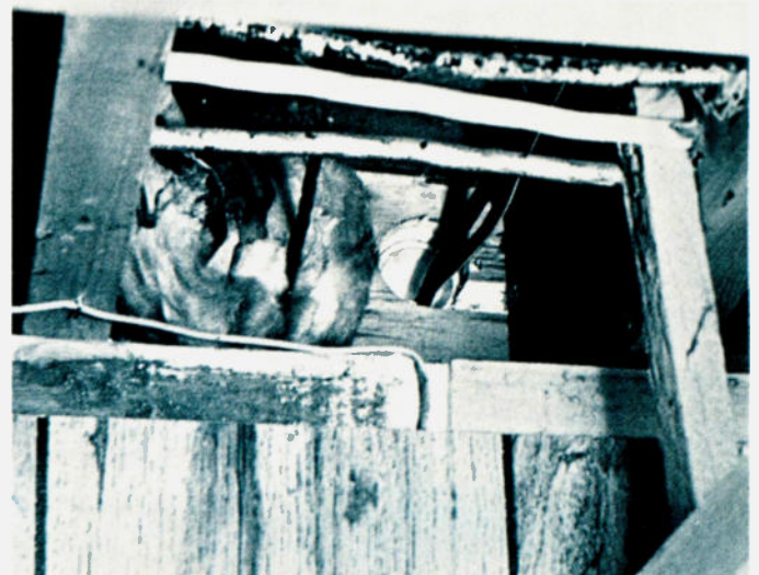
Inside-of-house view of the 90° elbow and the cables routed through it into the house.
