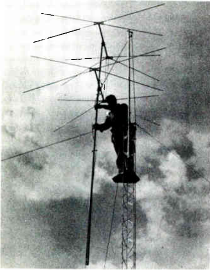
Installation of a television antenna and tower. The illustration shows the use of a platform, rope, and pulley. Note a safety belt is worn by the installer.
