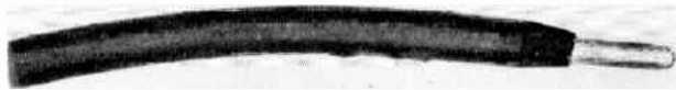
Fig. 14. The ends of insulated wires should be bared or "skinned" with tapering cuts, not square cuts.
