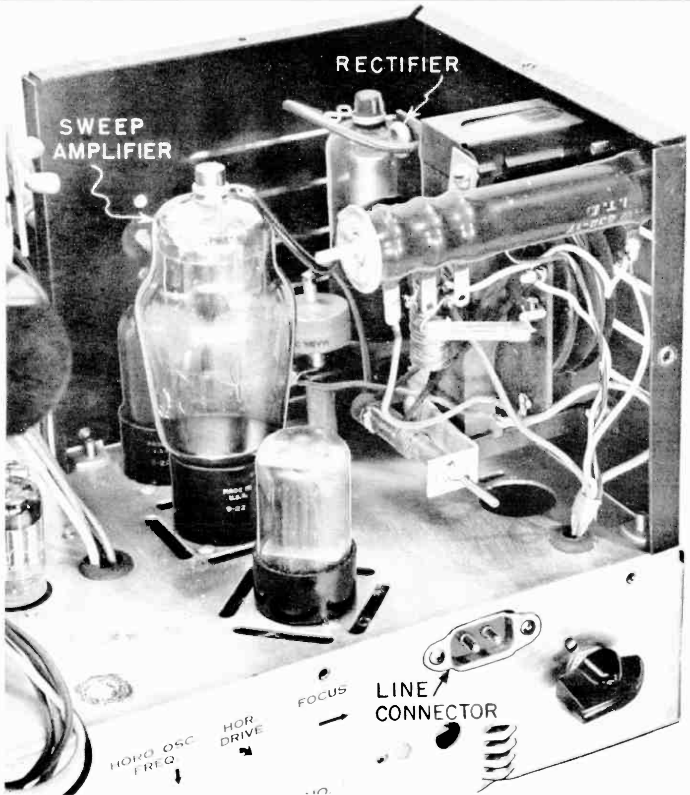
Fig. 10. Caps on the sweep amplifier and rectifier of a high-voltage power supply, also some of the other connections, will give painful shocks if touched.
