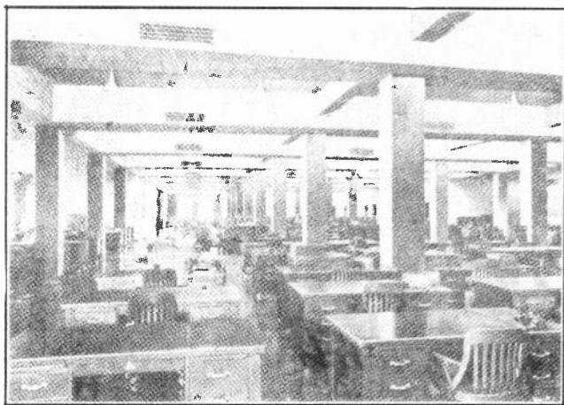
Fig. 12. Photo of the inside of a modern air-conditioned general office. Note the duct outlets along the ceiling beams. Much better efficiency and health can be maintained in such air-conditioned offices. Courtesy Jewell Tea Co.
