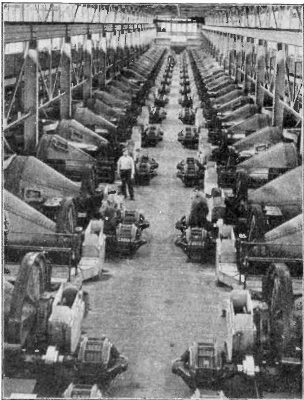
Fig. 13. This photo shows an installation of A. C. motors in a copper mill. Hundreds of thousands of motors in thousands of electrified factories and plants require the services of trained electrical maintenance men.
