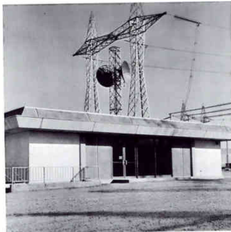
2—Pacific Gas & Electric Company's EHV intertie (top) has eight 500-kV substations, each monitored by a satellite computer. The system's central computer, located at the operation center, consolidates the substation monitoring and alarming and performs other super-
