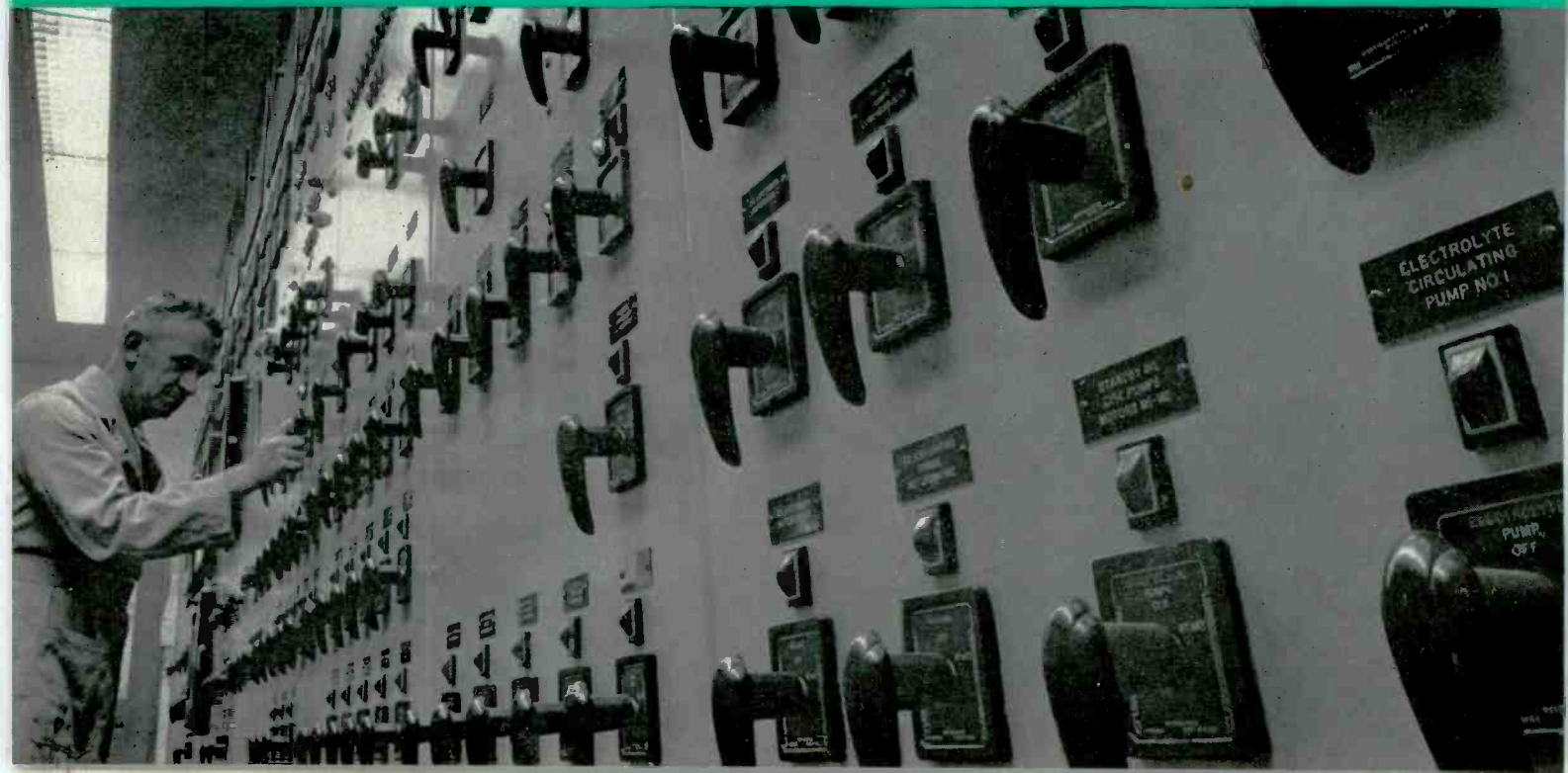
This array of controls is located in the motor drive control room, and is used to operate the four huge motors shown above.
