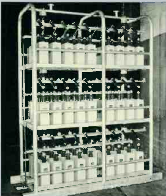
Fig. 10—This is a standardized open-type assembly of outdoor units. The pipe frame shields against corona.
