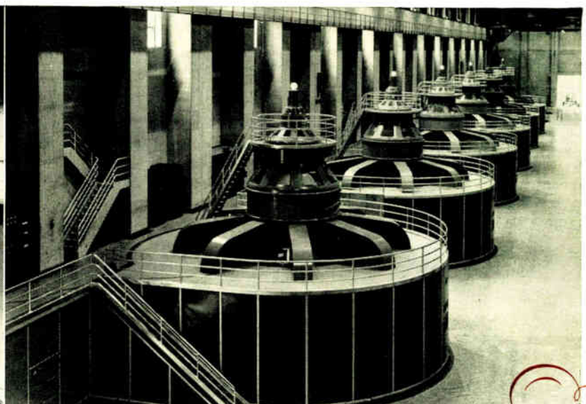
Installation of the 82 500-kva units (above) at Hoover Dam began in 1933. In each wing at Grand Coulee (left) will be nine, 108 000-kva, 120-rpm units all installed or under construction.
