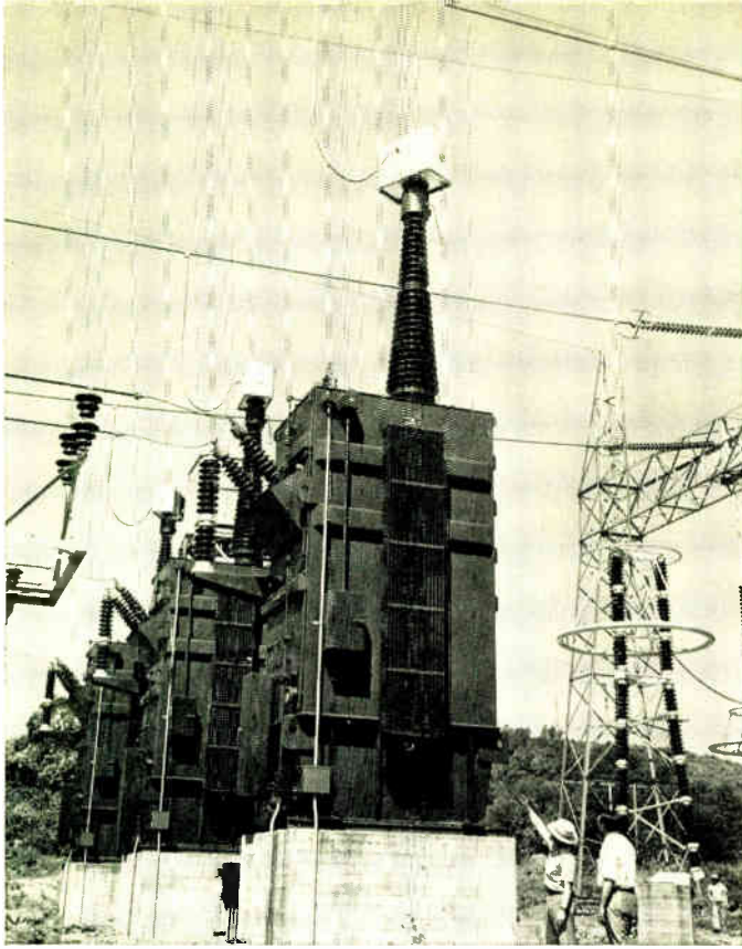
Here data is being obtained for construction of lines above the 287-kv limit. Shown are the 500-kv transformers and lightning arrester on the experimental lines at Tidd station.
