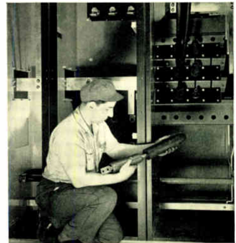
Fig. 12—Rear view of the metal-clad type of industrial-network load bus unit showing the limiter compartment.
