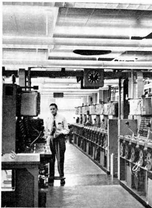
Figure 11. Fifth floor switching aisle at Portland, showing resilient cork flooring and fluorescent lighting
