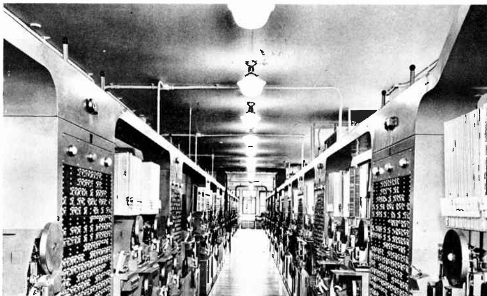
Figure 8. Special cable duct system—Atlanta reperfector switching aisle
