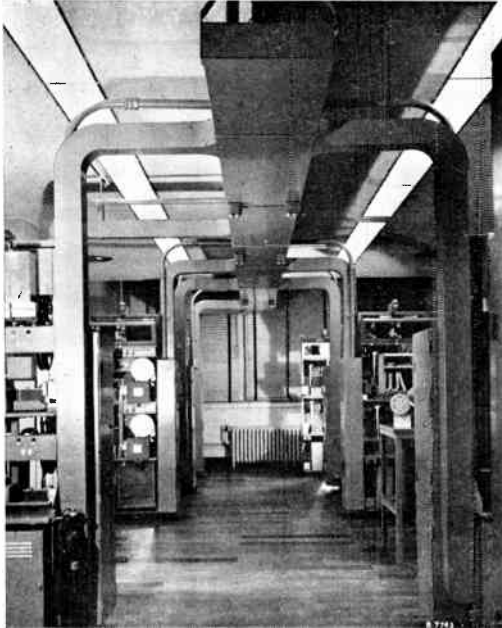
Figure 3. Overhead cable duct system— Philadelphia
