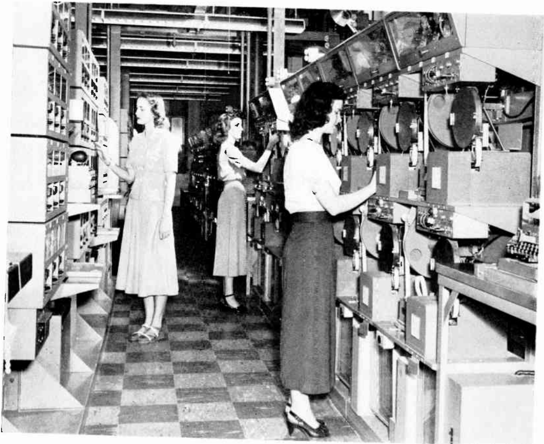
Figure 5—Modern selective switching reperforator installation
