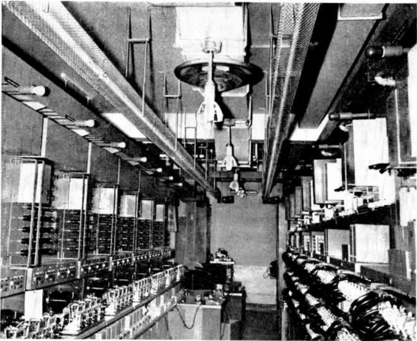
Figure 1. Switch room at Syracuse, N. Y., showing light beams of smoke detection system shielded by perforated metal cages
