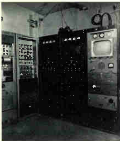
Figure 2. The KG2XDU transmitter racks.
