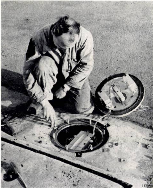
Fig. 13. Three transformers of the simplest type mounted in a flush runway light (as shown in fig. 21 of the article referred to in note 1 ). The cover, only the bottom of which is seen in the photograph, contains one omni-directional top light and two beam lights (one for each landing direction).
