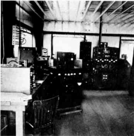
Figure 17. Interior of NBS Field Station Near Boulder, Colorado, Established to Monitor and Study the Signals Transmitted by Radio Station WWV and WWVH. The station is also used as one of the network of ionosphere probing stations maintained by, or operated in cooperation with, the National Bureau of Standards. The C3 ionosphere recorder (right, background) is one of the basic instruments used widely by science and the military for investigating the outer atmosphere by radar techniques.
