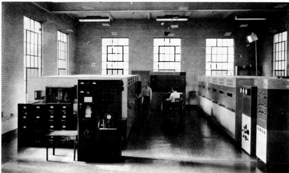
Figure 16. Interior of NBS Radio Broadcasting Station WWV. The banks of six transmitters are carefully monitored and precisely controlled to generate signals with an accuracy of two parts in 100 million.
