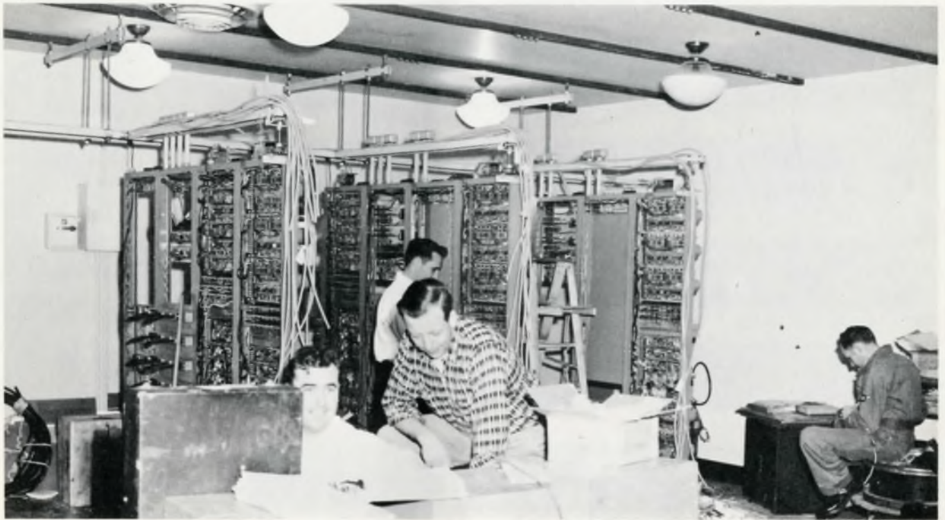
Installation Engineering personnel at work in the field, installing a Philco Microwave system for the Air Force.
