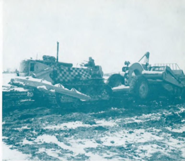
HUGE EARTHMOVING EQUIPMENT began work for Philco's Research Center. Thousands of cubic yards of earth had to be moved in preparation for the construction to follow.
