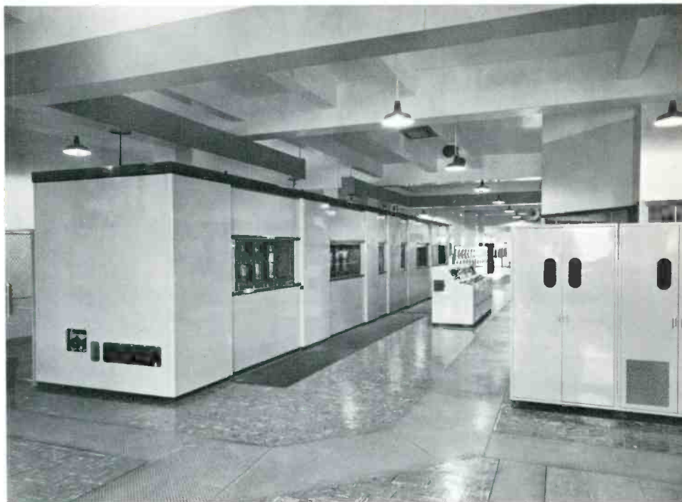
Figure 3 — Part of transmitter room of the VOA Philippines Relay Station showing Machlett ML-5682's in Continental 1 Mw medium-wave transmitter which broadcasts to Asia on 1140 kc.
