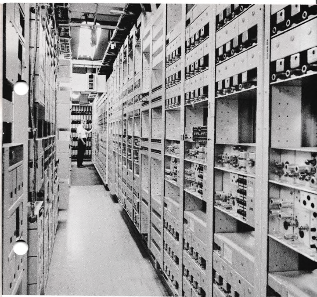
Figure 1. Carrier equipment like shown above enables hundreds of channels to be transmitted over a single radio beam. Increasing traffic density makes it imperative that some sort of standby protection be provided for microwave equipment.
