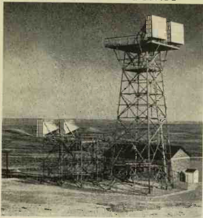
At Creston, Wyo., where the cross country TV system crosses the Continental divide, the microwave relay transmitting and receiving antenna are at different heights. Tele-Tech photo.
