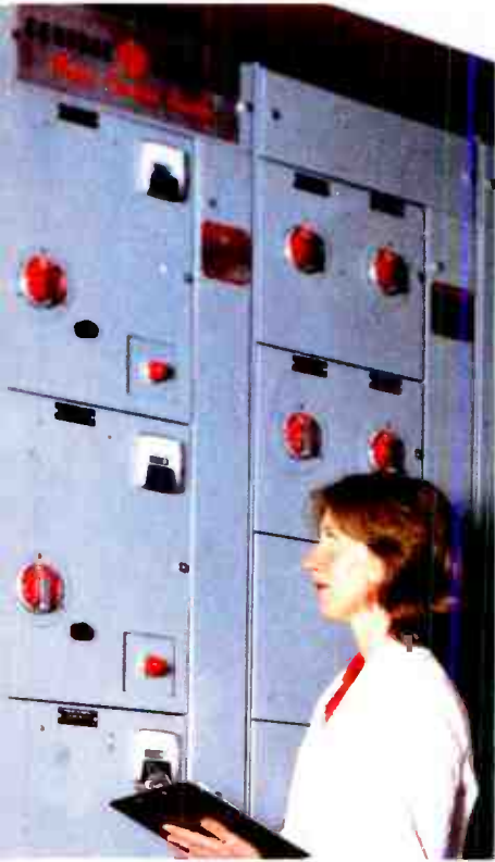
GE motor control centers regulate water treatment operations.
