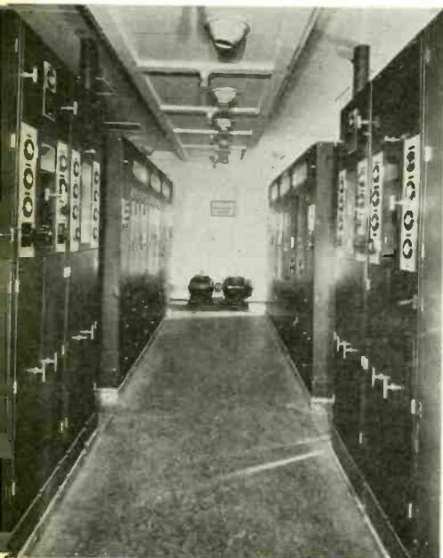
THE TRANSMITTING ROOM. ANOTHER VIEW OF THIS ROOM IS SHOWN ON THE FRONT COVER.
