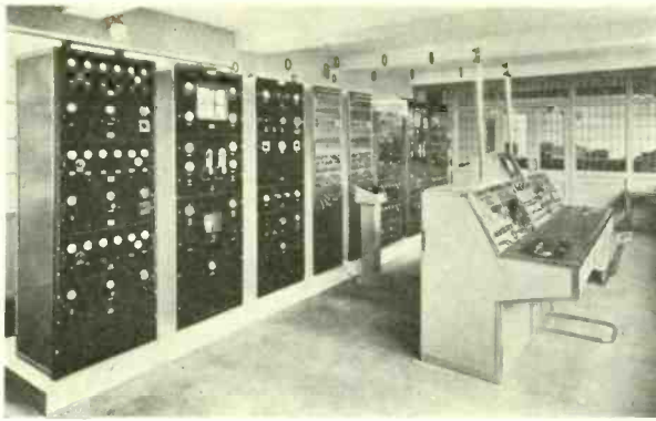
FIG. 6. EQUIPMENT ROOM IN HIGH-LEVEL STATION.
