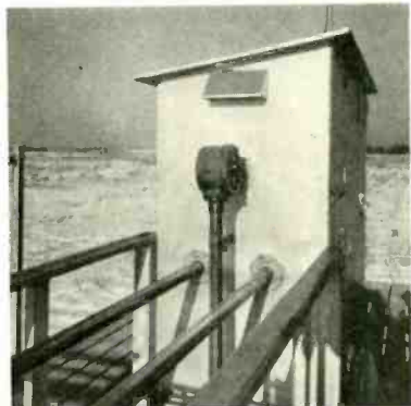
CENTER COUPLING HOUSE, MIDWAY BETWEEN THE TWO END TOWERS, WHICH CONTAINS THE PHASE SHIFTING AND TUNING UNITS. THE NETWORK THROUGH WHICH THE MAIN TRANSMISSION LINE DIVIDES THREE WAYS.
