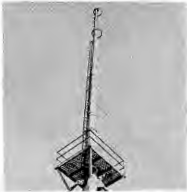
New two-bay G.E. f-m circular antenna recently installed by CBS atop 700-foot building at 500 Fifth Avenue, New York City.
