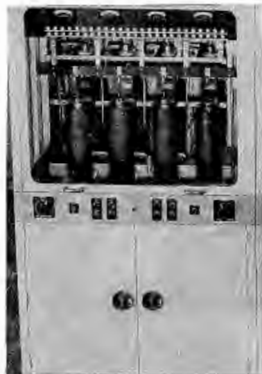
Figure 17 The rectifier cabinet.
