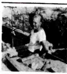
The author during construction of the ducts. The openings or ducts may be seen inside the manhole between the bracing.
