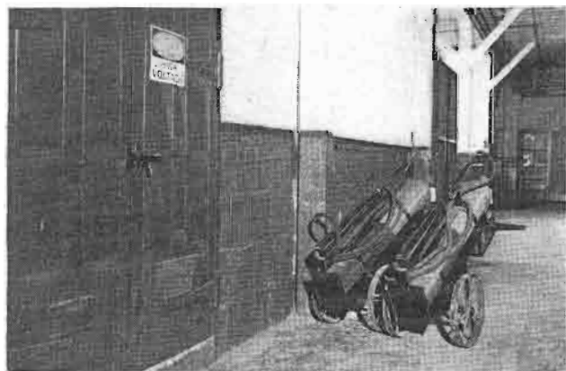
Two wheeled extinguishers (50 pounds capacity) at power transformer vault in RCA Camden plant.
