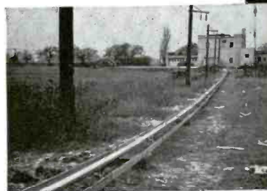
Below: A view of the installed line leading from the transmitter to WTAM's tuning tower.
