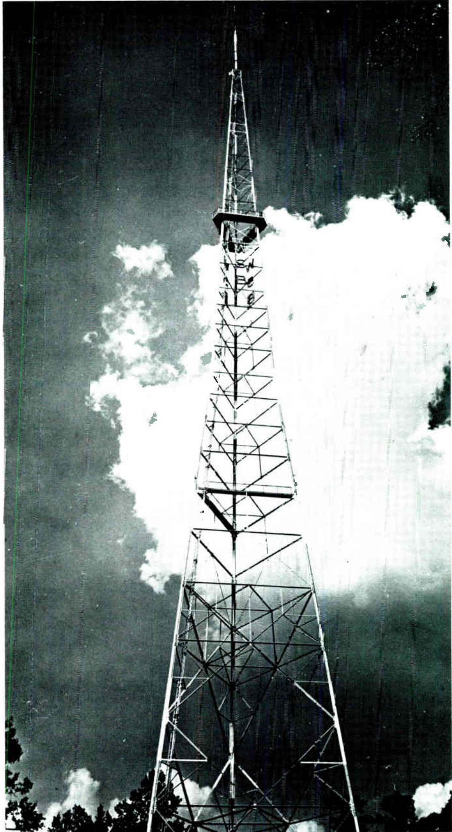
Station WSB's triangular self-supporting tower rises skyward to support a pylon antenna. Such towers are recommended where sites are in congested areas or where a tower is designed for erection on a roof-top.
