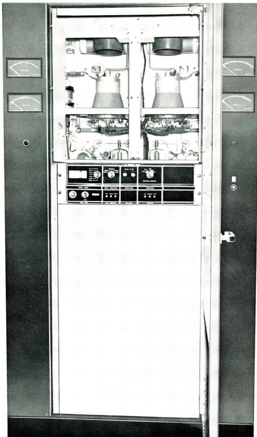
Front section of the exciter-modulator containing all components from oscillator through the driver stages.
