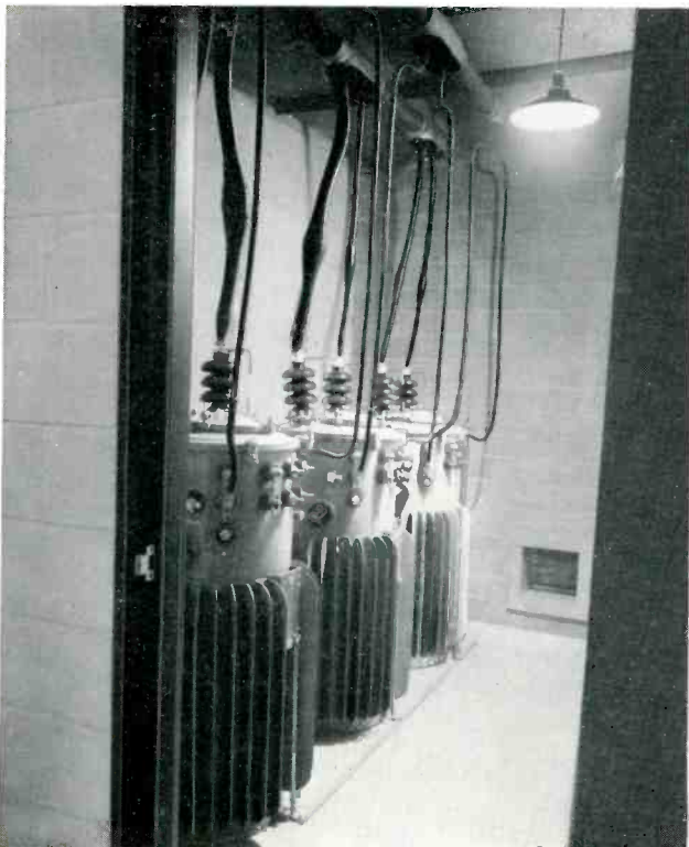
High voltage plate transformer vault.
