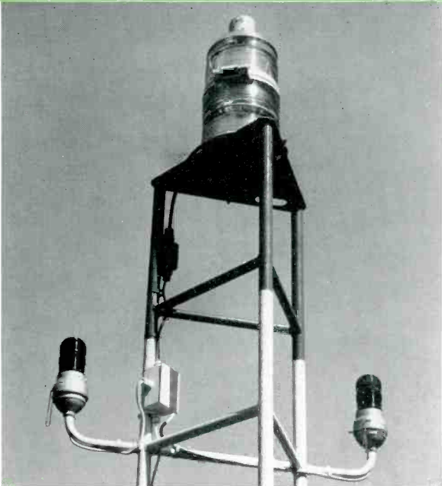
Main beacon and side obstruction lights shown powered by use of either lighting transformer or lighting choke coil.
