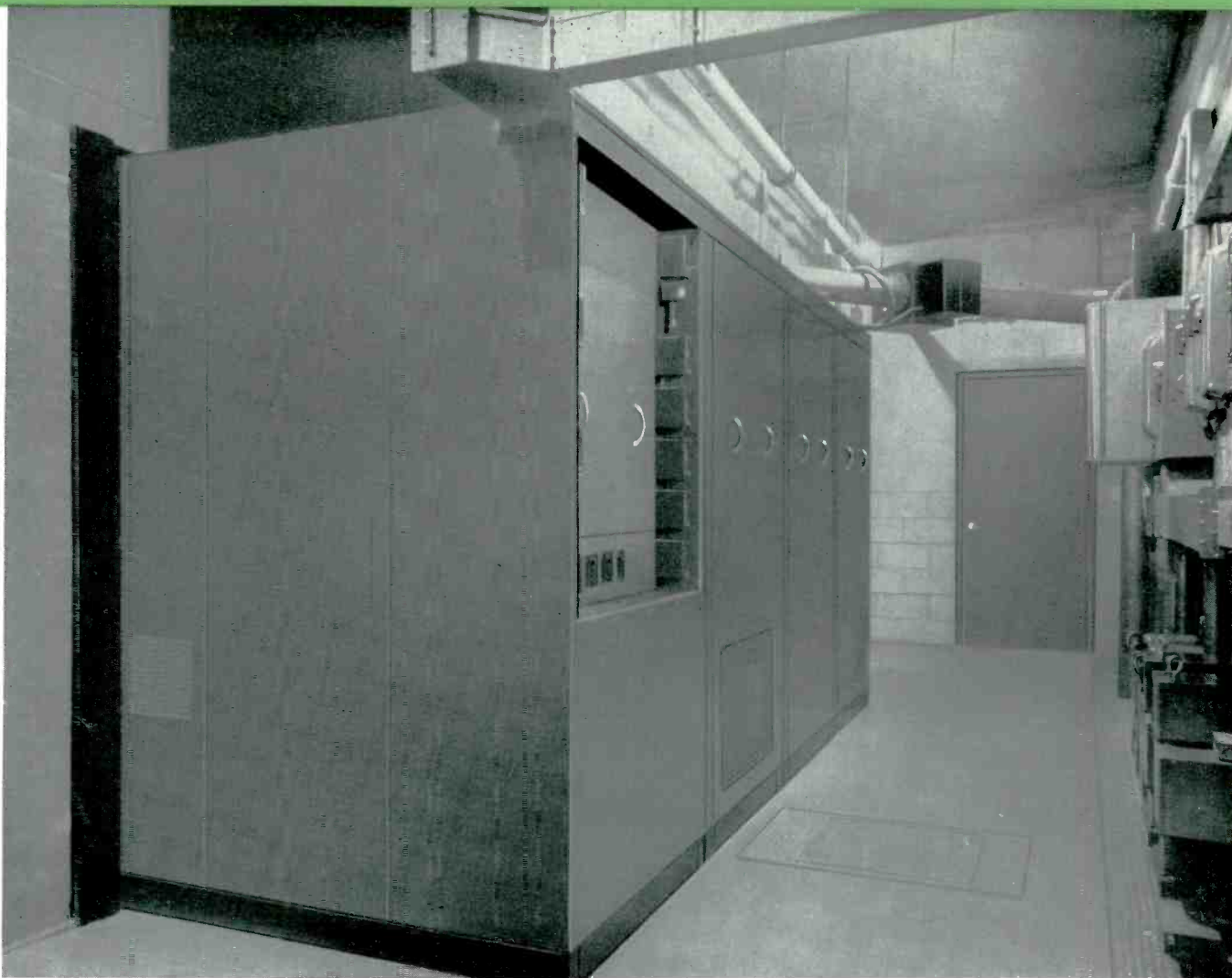
Rear view of the BTA-50G "Ampliphase" AM Broadcast Transmitter.
