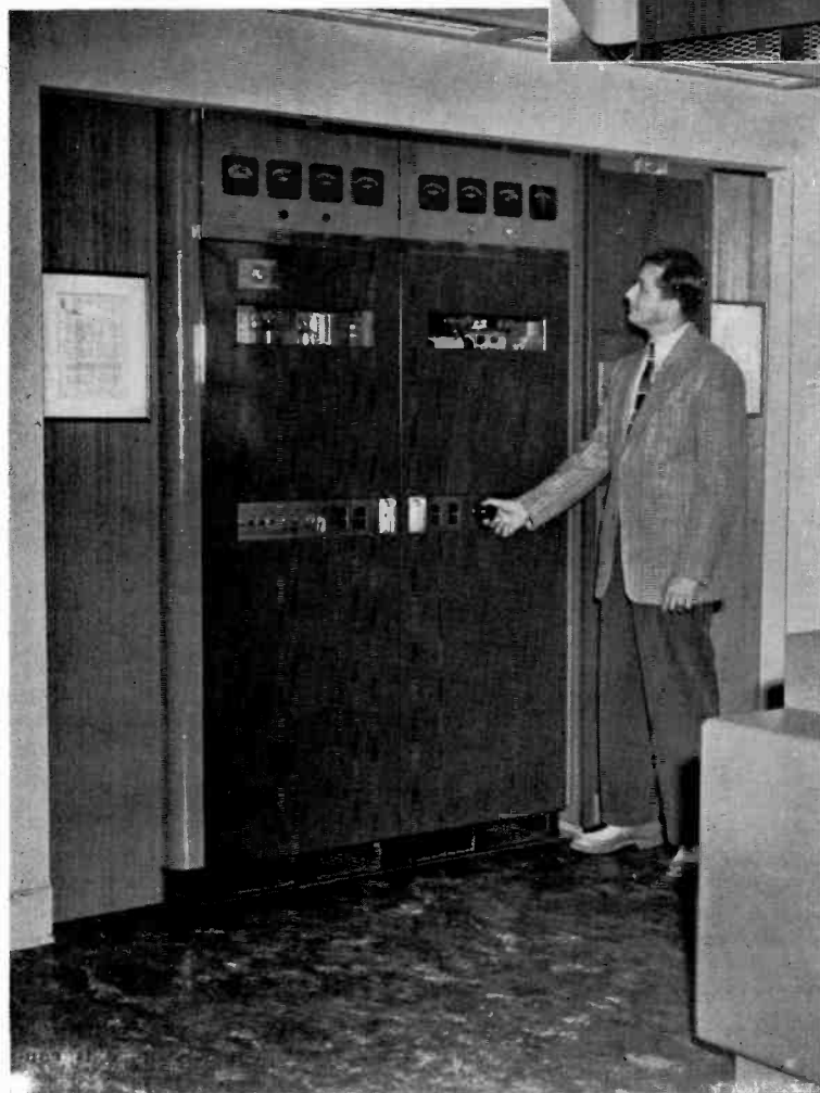
One kilowatt FM transmitter, Type BTF-1C, as installed at radio station WBRE-FM, Wilkes-Barre, Pa.
