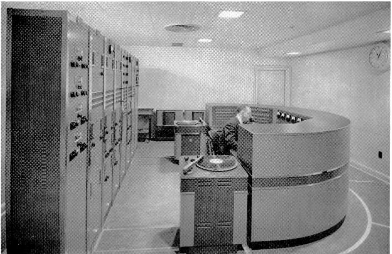
A completely RCA equipped master control console and associated audio equipment installed at WFAA, Dallas, Texas.
