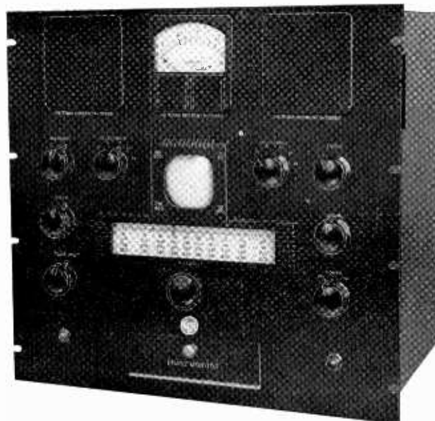
Remote Meter Panel
