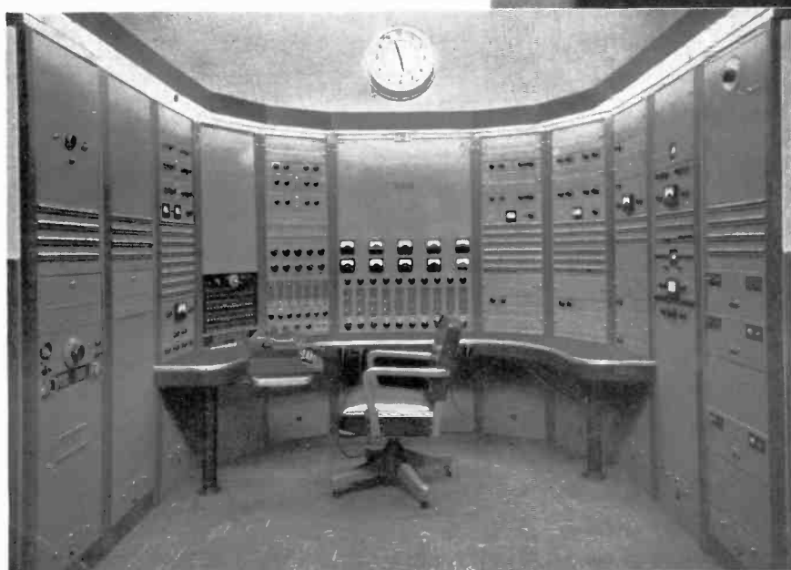
Deluxe, custom-built installation, com- pletely RCA equipped, at WNEW, New York City.
