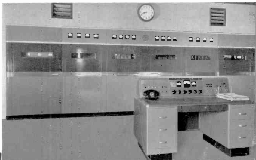
Installation of five kilowatt transmitter, Type BTA-5F, at KGKL, San Angelo, Texas. View shows left and right wing extension cabinets which contain broadcast audio and antenna phasing equipment.
