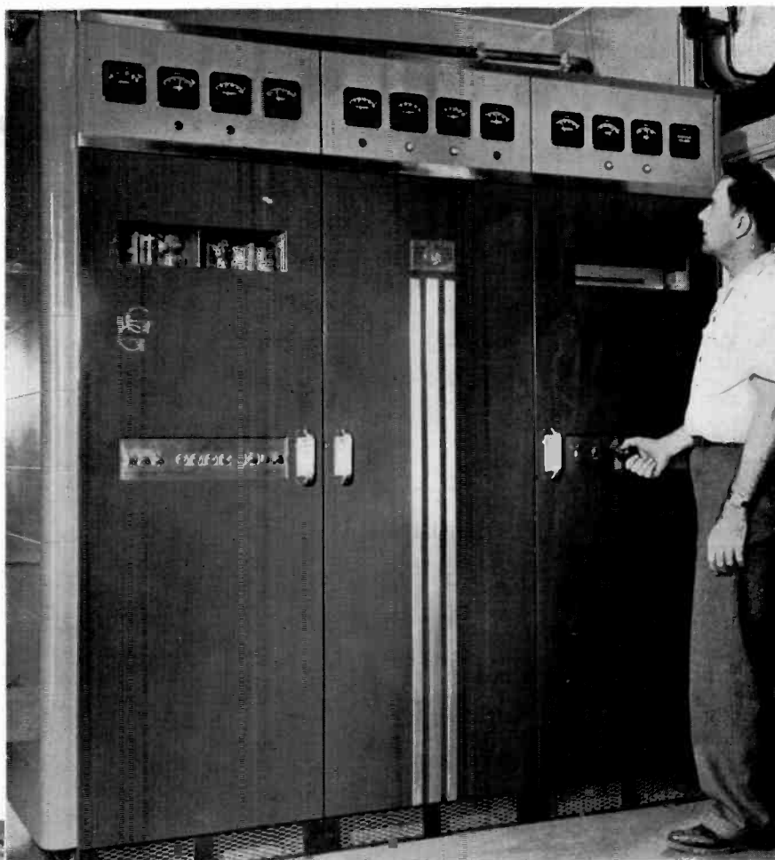
Adjusting line voltage on the three kilowatt FM transmitter, Type BTF-3B, at WCPA-FM, Bethlehem, Pa.
