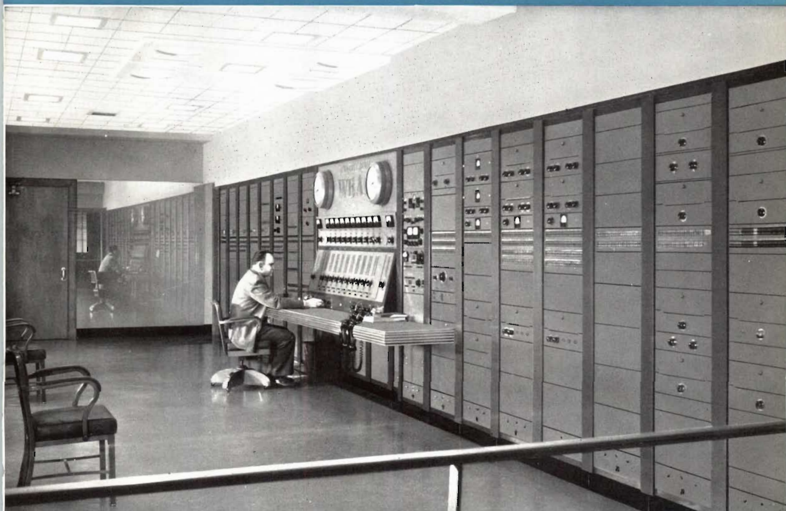
WBAP, Fort Worth. The master control installation pictured here includes 16 deluxe audio equipment racks. These are just part of WBAP's modern six-studio layout. The master control installation features an "In-Line" design for handling 16 inputs and 10 outgoing channels.
