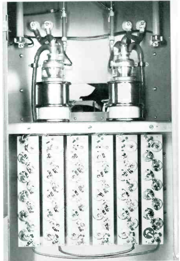
Modulator tubes and silicon high voltage rectifiers with cover removed.
