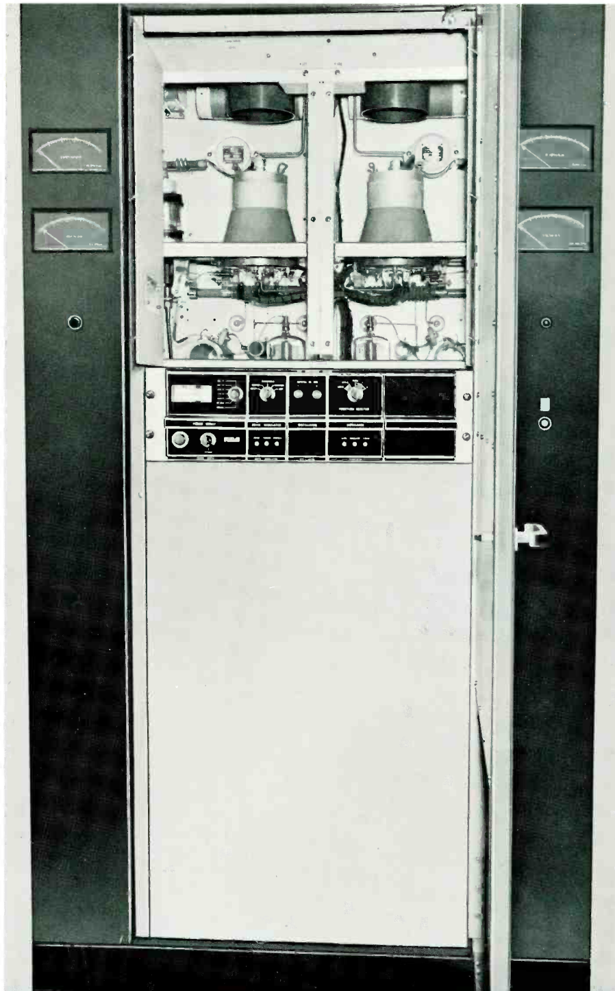
Front section of the exciter-modulator containing all components from oscillator through the driver stages.
