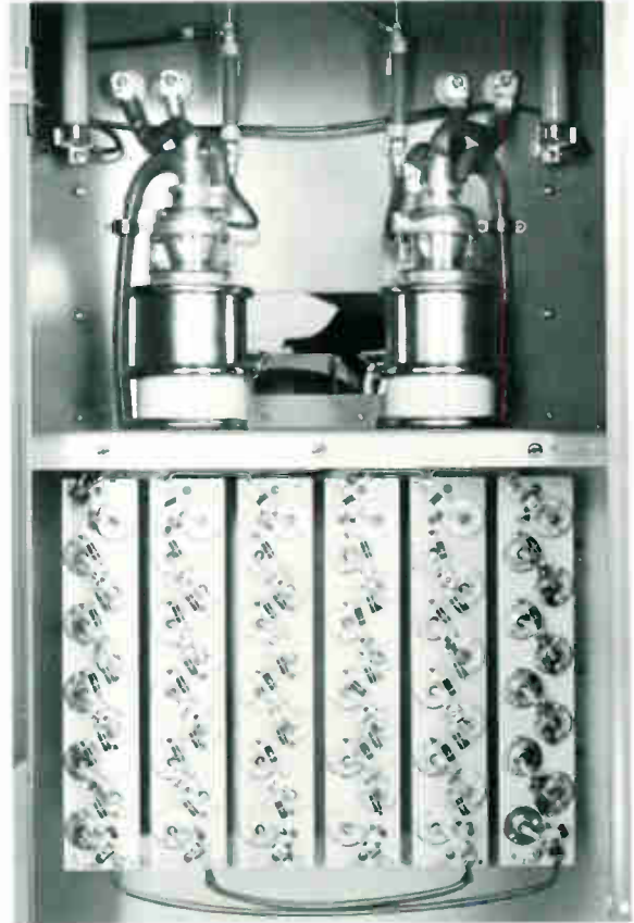
Modulator tubes and silicon high voltage rectifiers with cover removed.
