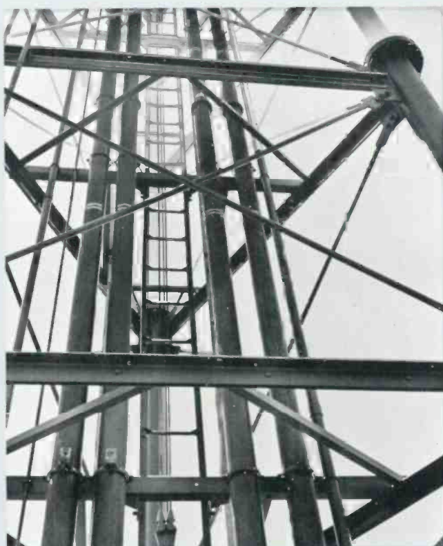
By placing a service ladder within the tower, the lattice braces form a safety cage for the servicemen.
