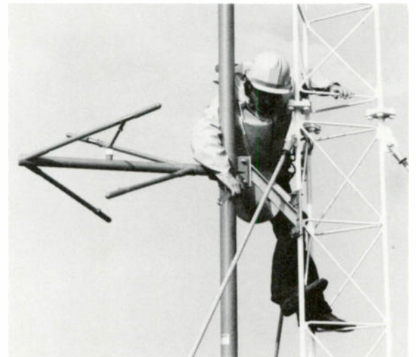
Rigger assembling JSCP antenna. Antenna assembly is quick and simple via EIA flanges, with the antenna bolted directly to the mounting bracket for maximum rigidity.
