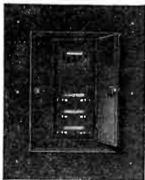
Small Door Open, Giving Access to Switches
