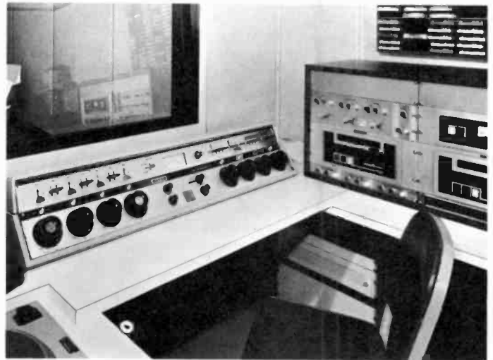
GATESWAY II CONSOLE AND CARTRIDGE TAPE EQUIPMENT WEEL, BOSTON
