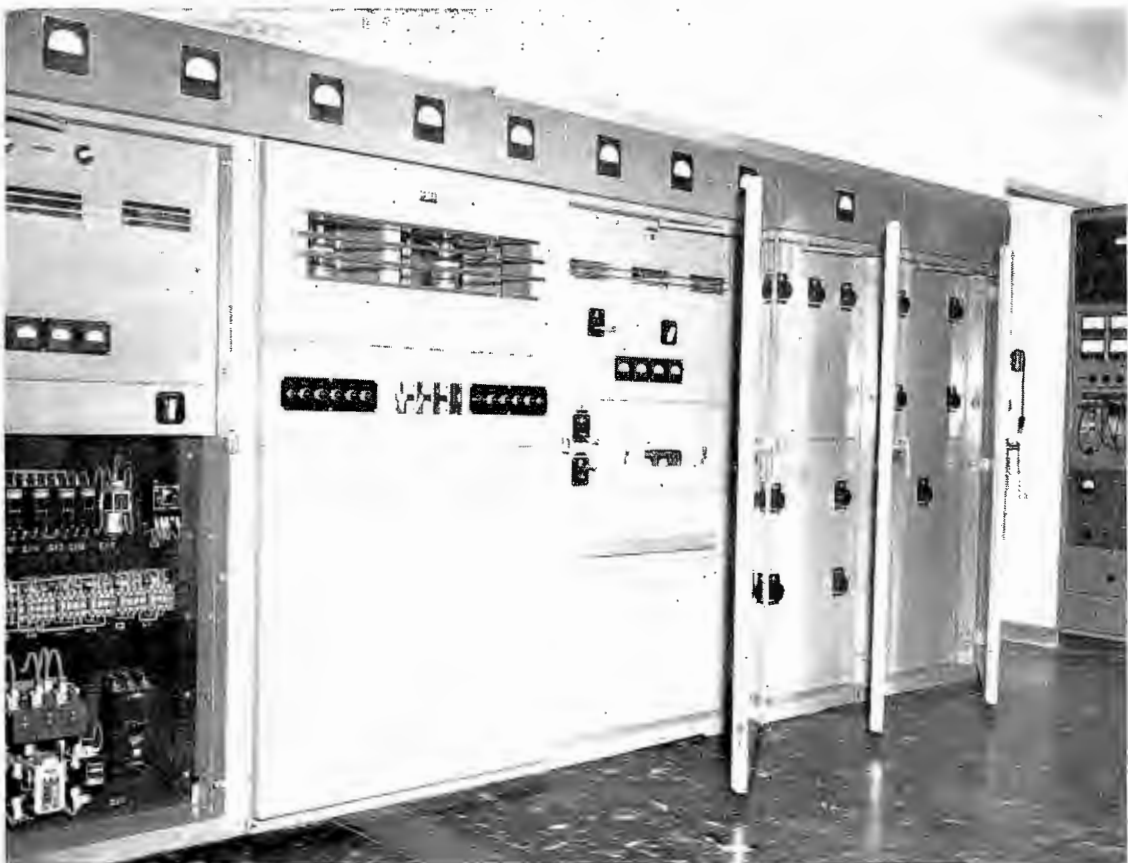
Below—Gates BC-5B 5000 watt equipment with five tower phasing equipment in matching cabinet at WENE, Endicott, N. Y.
