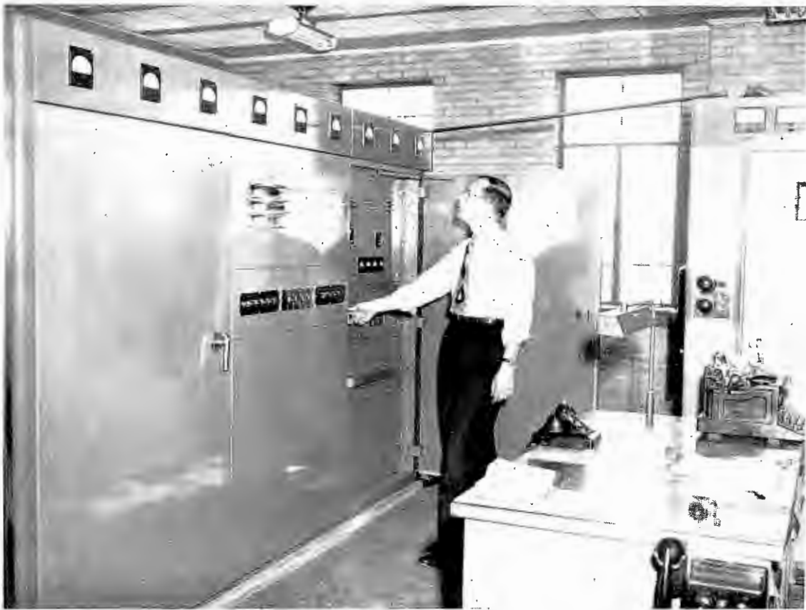
Above—BC-5B 5000 watt Gates broadcast transmitter installed at Radio Station WTAD, Quincy, Ill., CBS outlet and pioneer midwestern station.
