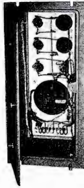
Above are front, internal and rear views of the rack mount, power supply part of the SA-40 equipment.
