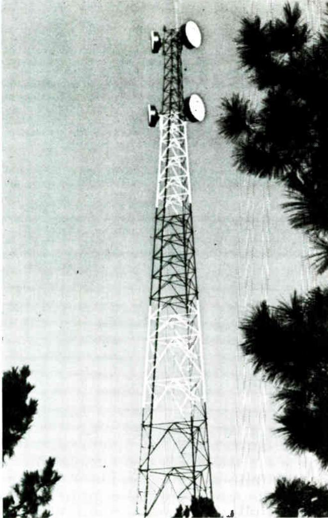
SSV SELF SUPPORTING TOWER
